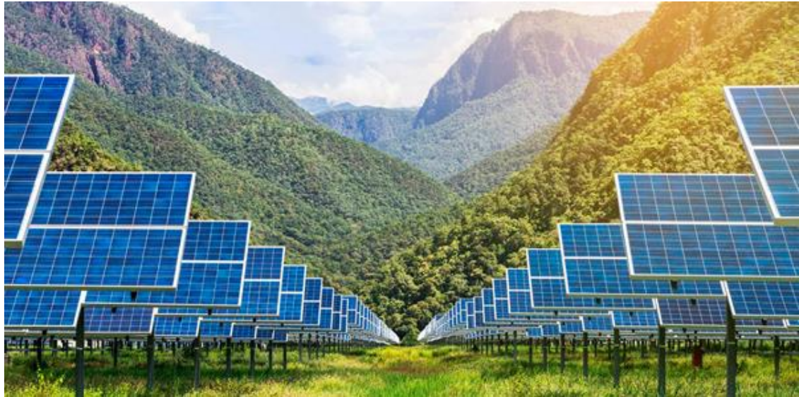
Picture 1. Layout view of solar power plants (SPP) in the Nagorno-Karabakh region.
